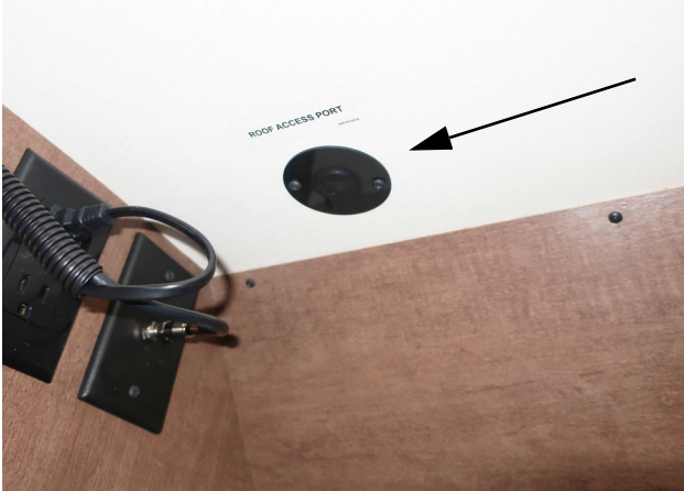
Roof Access Port (Located inside galley overhead cabinet behind TV) -Typical View
